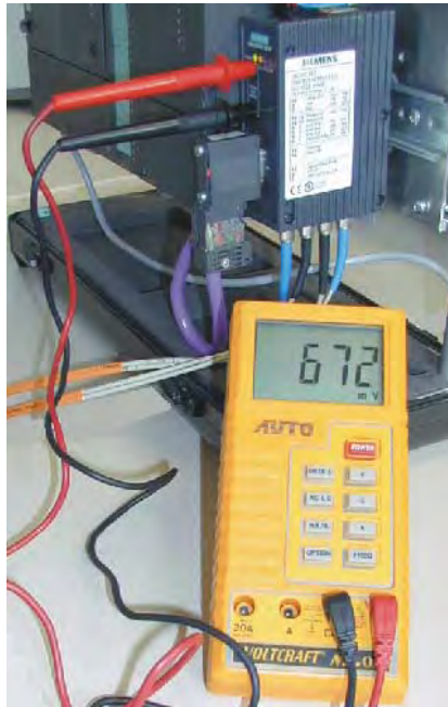
Figure A-6 Testing the Signal Quality on an OLM V3 with a Voltmeter
